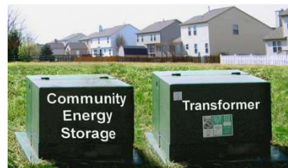
AEP Battery Storage Systems
